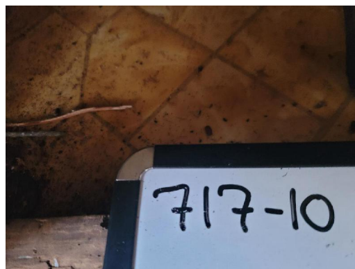
717-10 Rolled Flooring/Yellow (15% Chrysotile) Interior North Bedroom Closet (Appx 12 sq ft)
